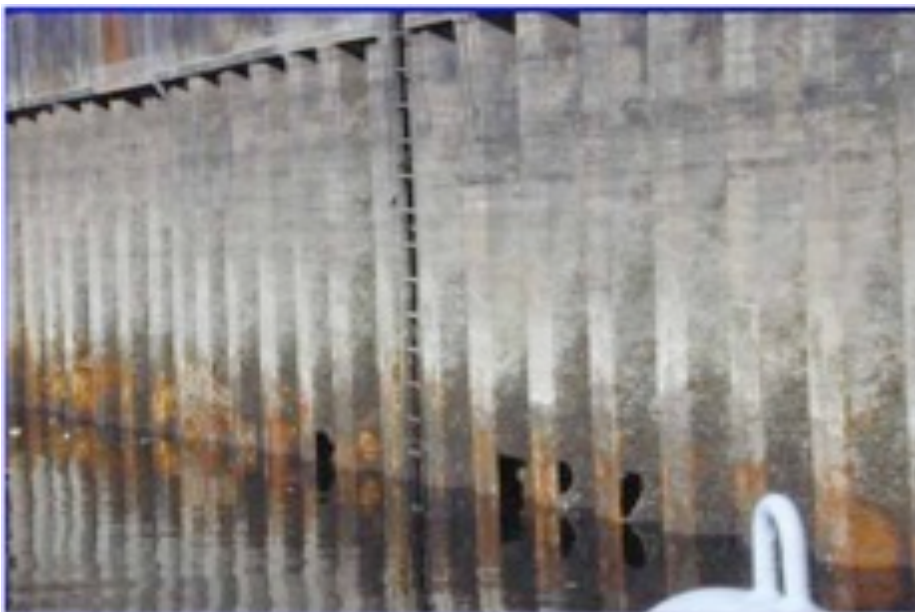
Figure 21: Low water zone corrosion of sheet pilings. 29
