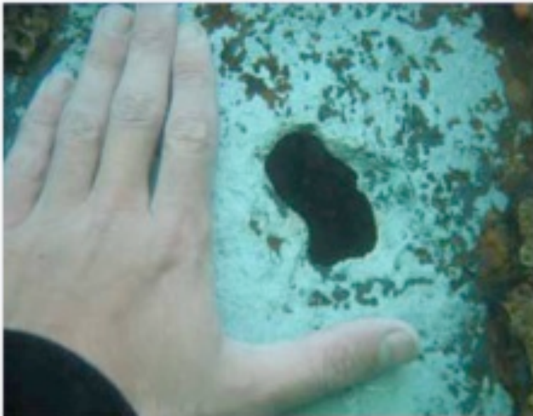
Figure 22: Pitting and wall perforation of steel piles by MIC. 28
