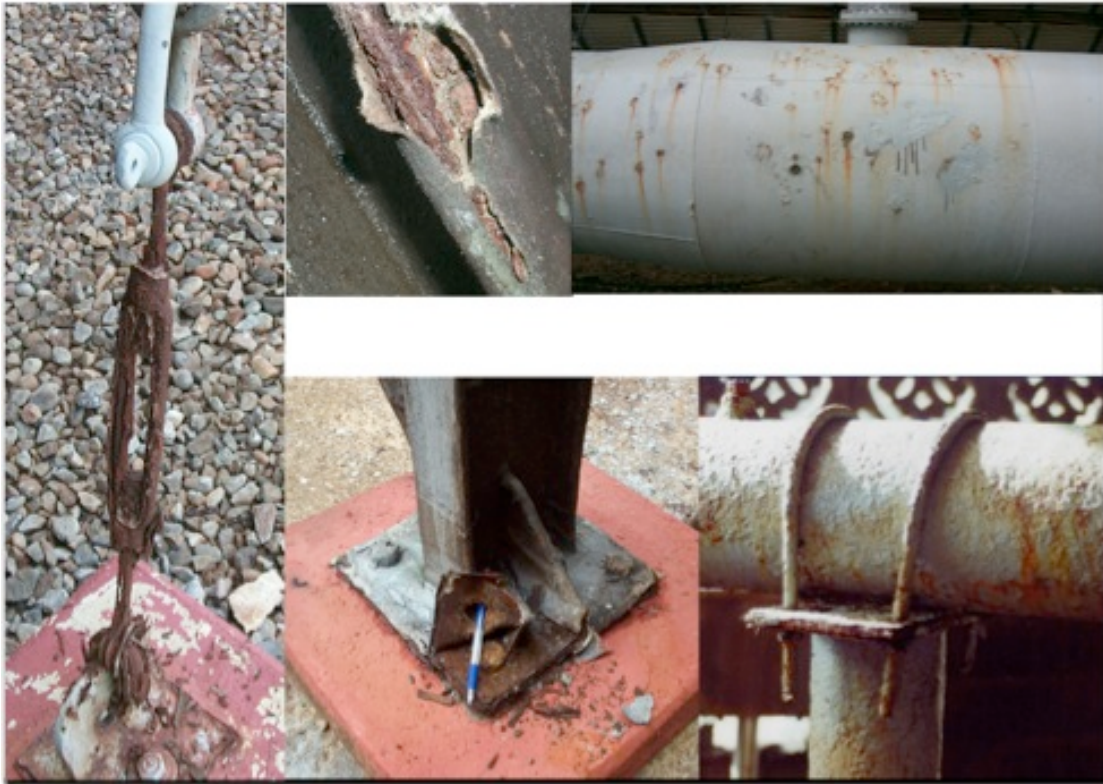
Figure 17: Corrosion of structural materials due to highly corrosive atmosphere in range of the plant. 26
