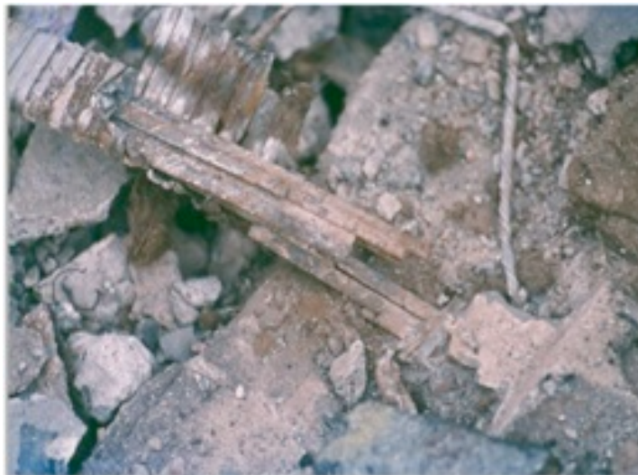
Cause of the collapse: stress corrosion cracking of prestressed steel in ring beam joint.
